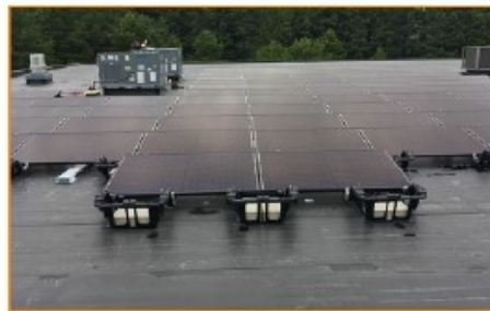
All wiring managed under module, FR510 chassis or in listed raceway.
