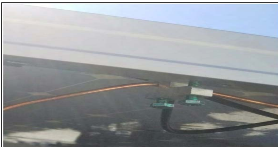
Figure 7- FR-SGB-4 Grounding Lug
