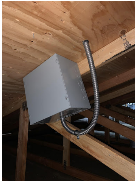
Figure 35. Conduit to Attic Enclosure
