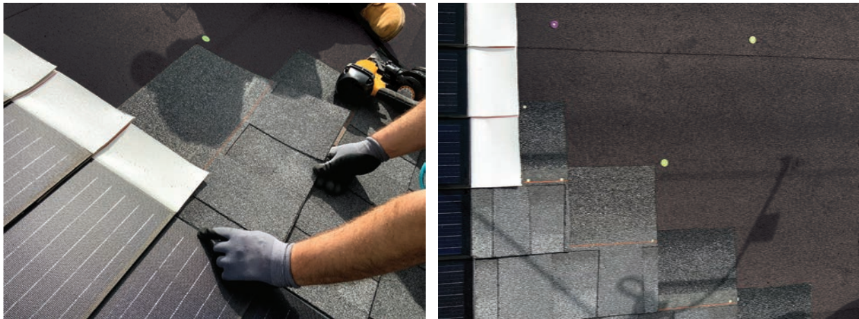
Figure 28. Shingle offsets on right edge of array
