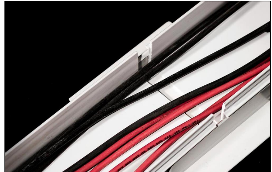
Wires in RayTray
