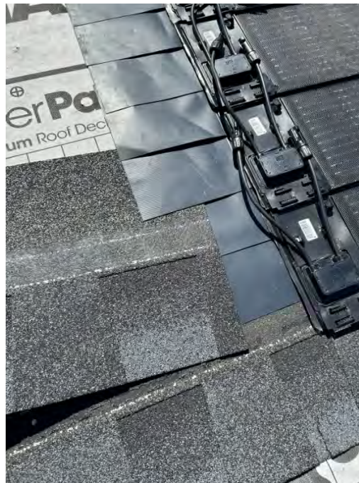
Figure 35. Shingles on the left edge of the array
