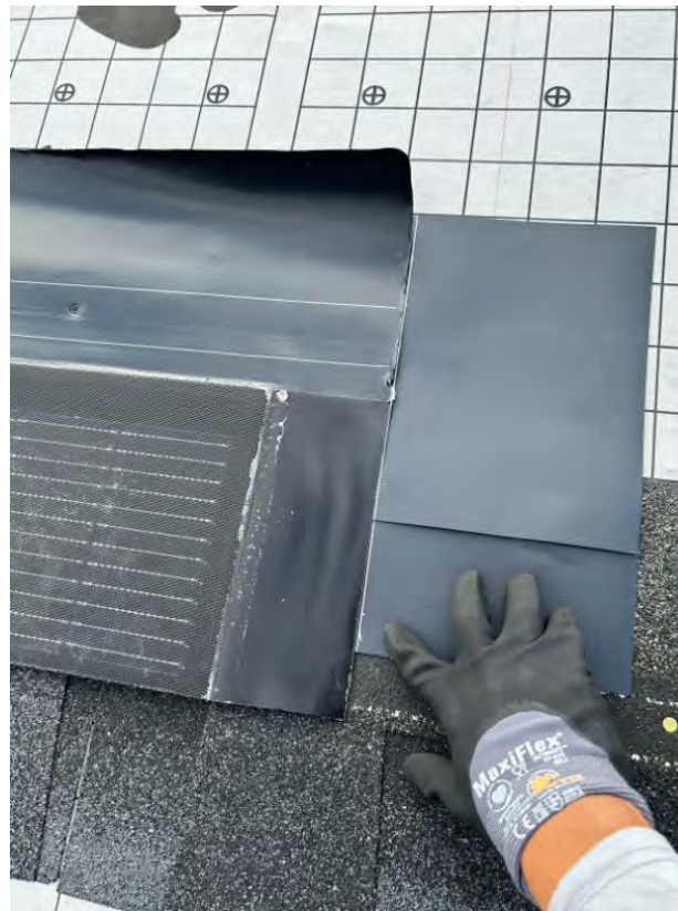
Figure 29. Step flaps going up the right side of a column
